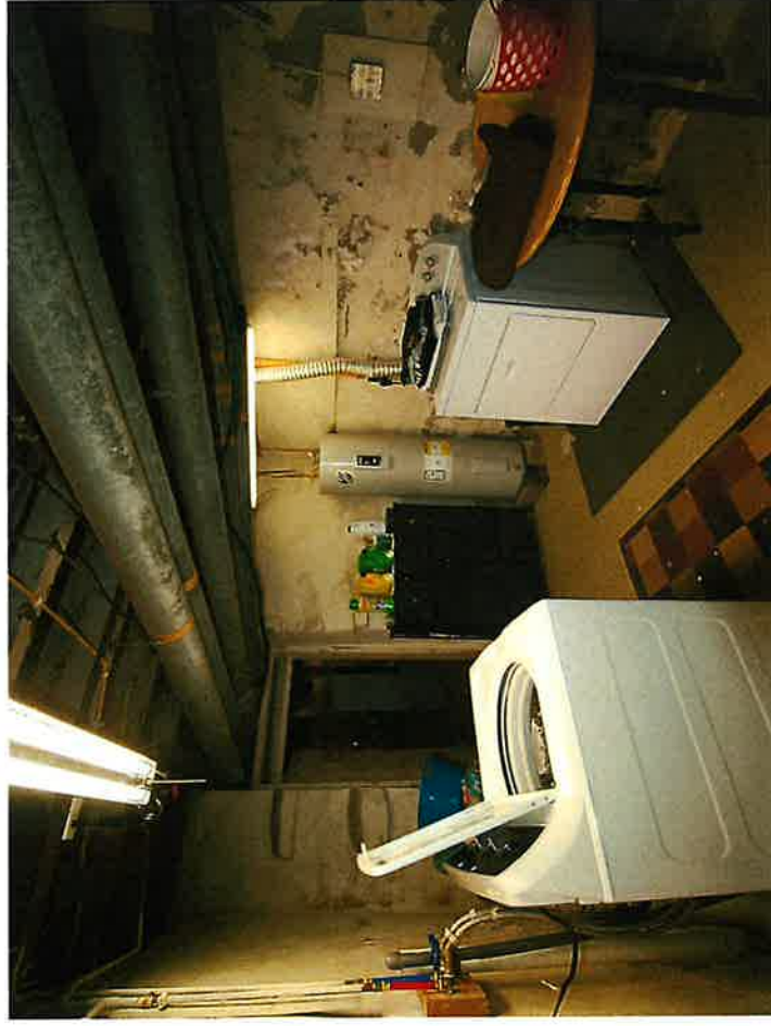
Functional laundry space with utilities
